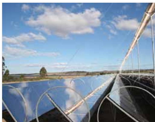
Concentrated Solar Power
